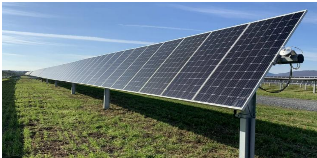
14MW Hy-Grid Solar System
