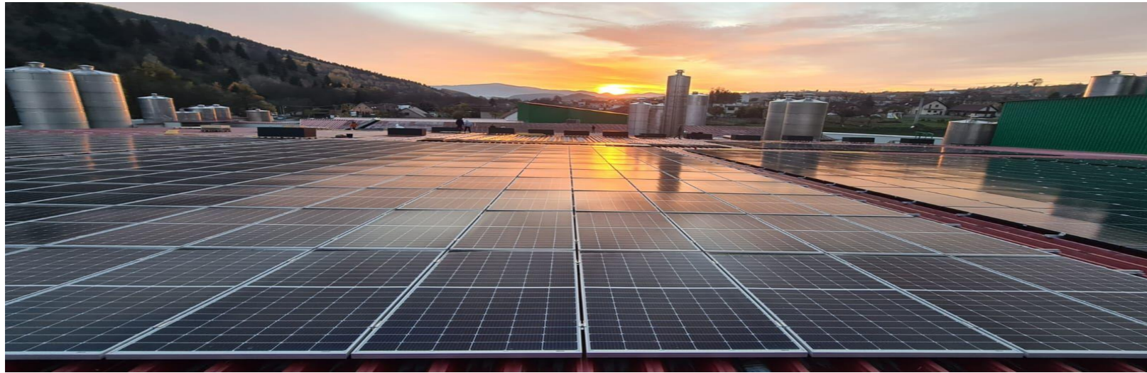
20MW Hy-Grid Solar System for Oil & Gas project
