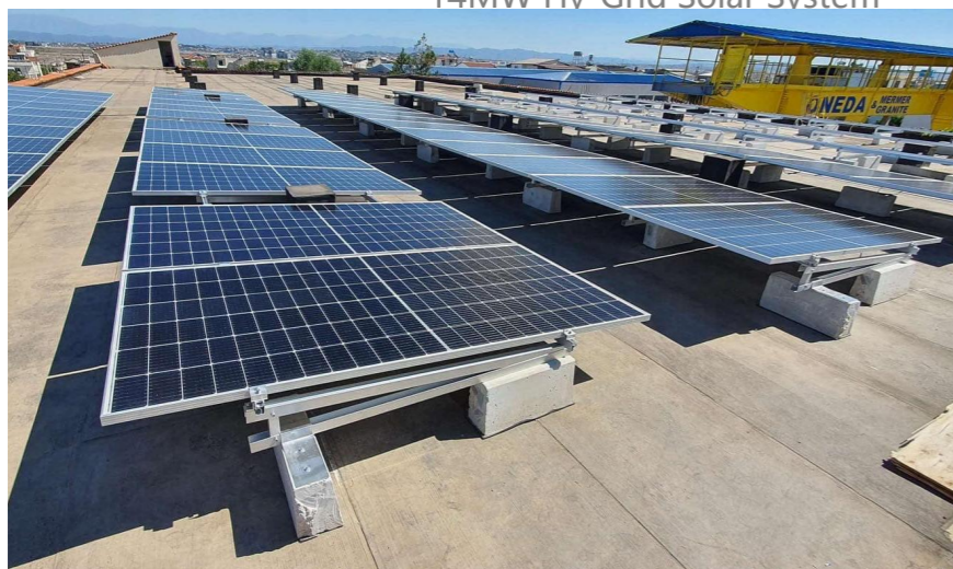
2MW On-grid Solar System in Hungary
